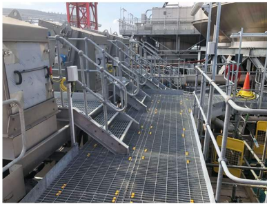
Steel grating platform mezzanine
