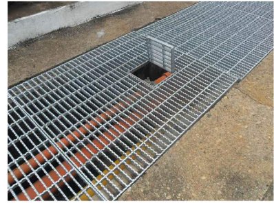
Steel grating trench covers
