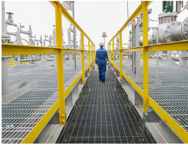
Steel grating platform walkways
