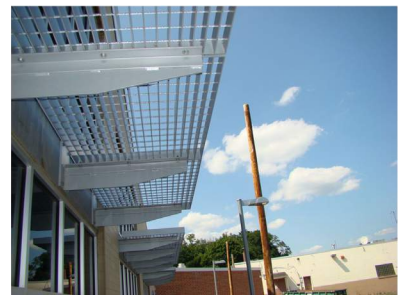
Steel grating sun shade panels
